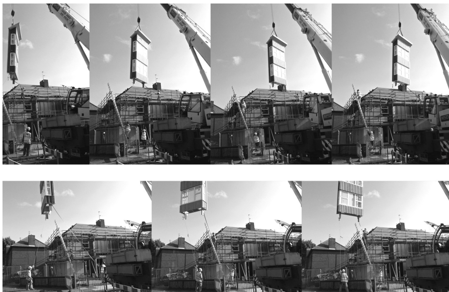
Figure 3. The Walker Garden Suburb project, in the east end of Newcastle upon Tyne: installing one of a pair of two-storey bay windows manufactured off-site. With one window, installation was done while the home in question was still being occupied; with the other, the premises were vacated for five weeks. These new, large bay window units made for increased energy efficiency
