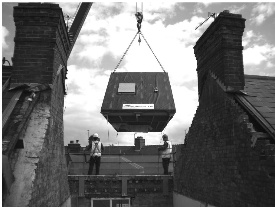
Figure 1. Project Cottesmore, Leicester: installing a roof pod manufactured off-site. Earlier retrofitting of the house to a low-carbon specification had led to the extensive use of bulky internal insulation materials, and so to unfortunate reductions in room size and available space. The roof pod compensated for this loss of space, and exemplifies the social factors that must be taken into account in any quest for residential energy efficiency
